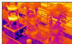
Electric Equipment Inspection
