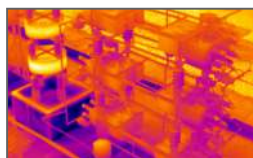
Electric Equipment Inspection
