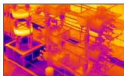
Electric Equipment Inspection
