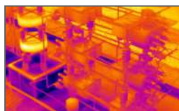
Electric Equipment Inspection
